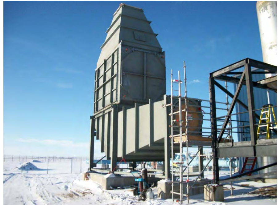
Waste Heat Oil Heater ("WHOH")
